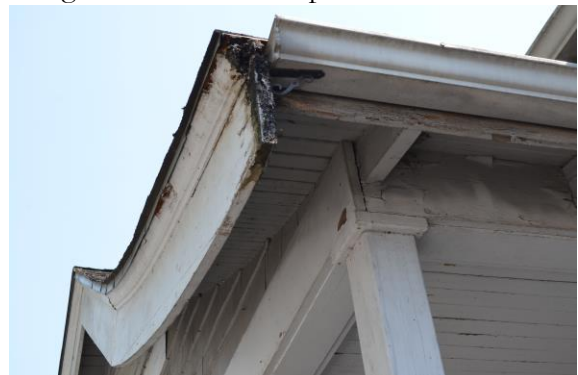
Before: Dry rot along fascia
