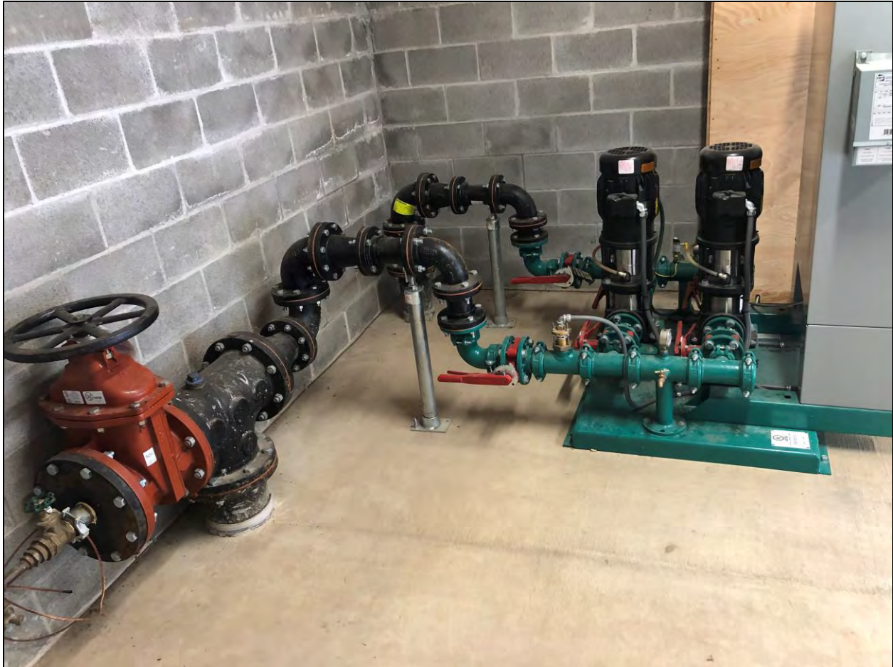
FIGURE 3-7: ELK RIDGE BOOSTER STATION
