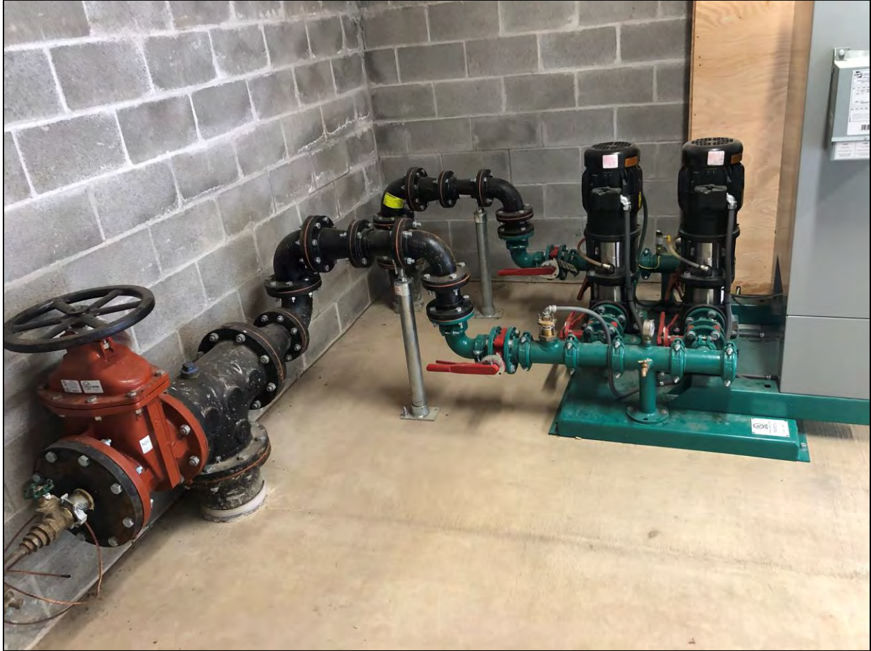
FIGURE 3-7: ELK RIDGE BOOSTER STATION
