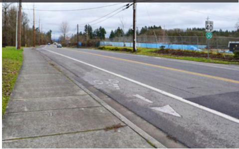
Curb-tight concrete sidewalk and bike lane on Old Portland Road looking north
