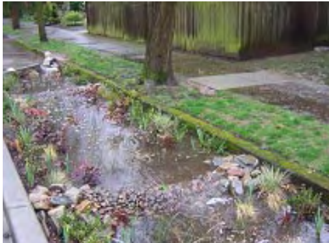
Swale retaining rainwater after a storm event
