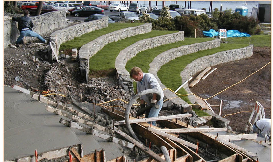
Volunteers, in a partnership with the City of St. Helens, constructed the amphitheater used as seating during community events.
