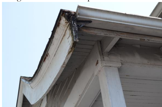
Before: Dry rot along fascia
