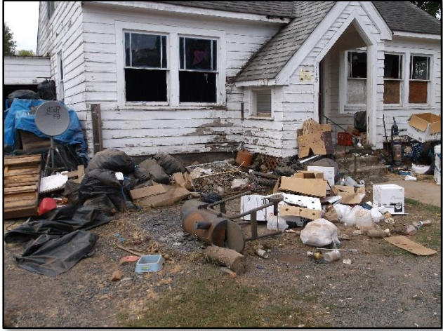
The residence at 115 South Vernonia Road prior to a Code Enforcement response in the summer of 2015
